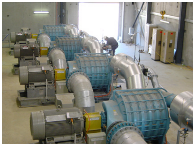
Installed in process industry
