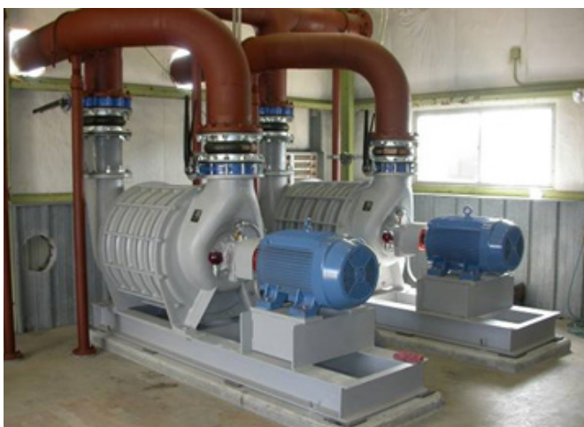
Installed in wastewater industry
